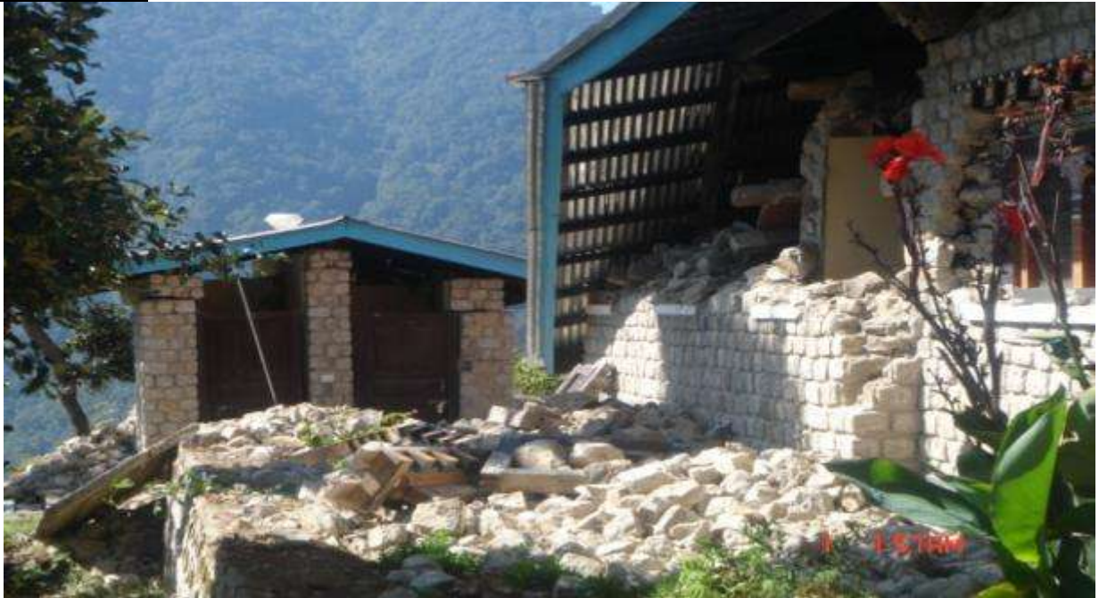
The Narang BHU Grade II buildings completed in 2007, consist of 4 buildings which have collapsed due to the quake.
