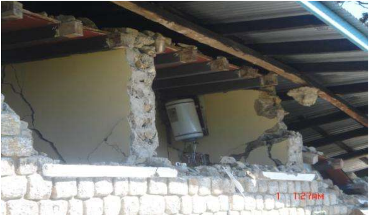
No proper joints between walls
